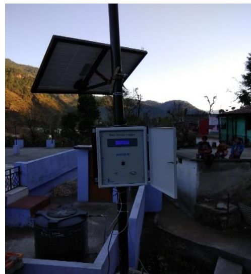
Rain gauge Station installed at (Siso)
